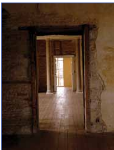
Layers of history and restoration at an Elizabethan country house: Kirby Hall, Northamptonshire.
